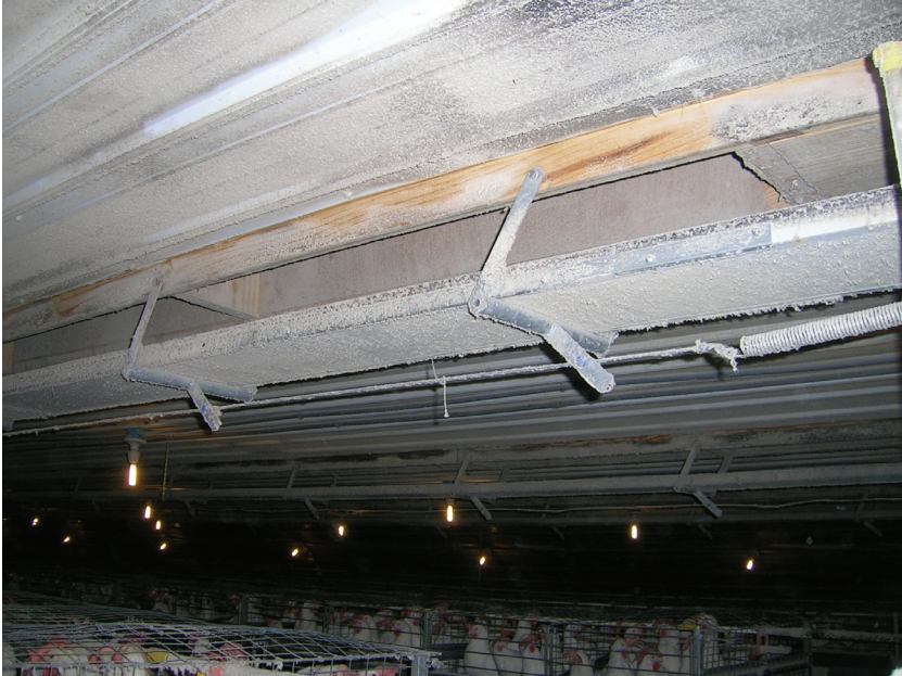
Fig. 5. Horizontal baffle with inlet slot above it is adjustable to match inlet area to air flow capacity of operating fans.
